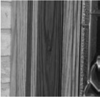
Figure 25: Holes must be filled and painted over to prevent jambs from cracking and/or peeling. (Very Important)
