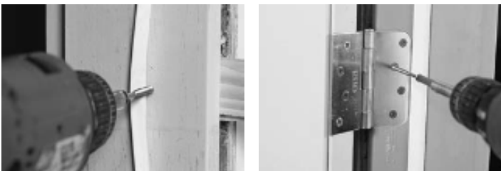
Figure 21 and 22: The second set of supplied screws is installed in the vacant hinge holes or under the weather-stripping.
