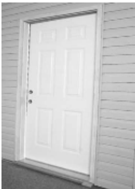
Figure 9: Gaps are seen at the top of the door unit
