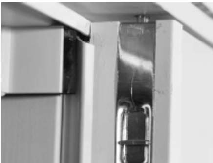
Figure 17: Correct sagging until the flush bolt slides freely into the pre-drilled hole in the head/threshold.
